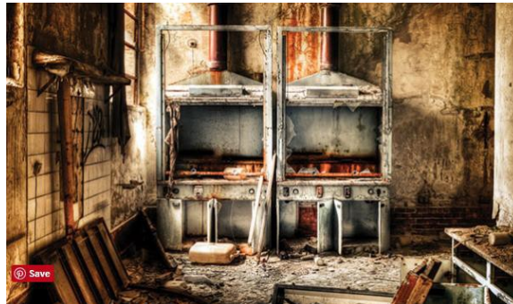
Laboratory fire as a result of improper use and storage of flammable liquids.
