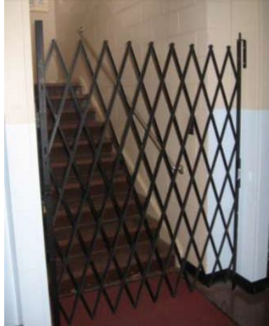
Locked gate obstructing a safe exit from a stairwell.
