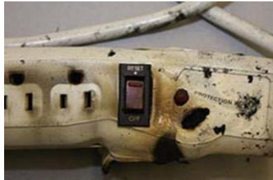
Overloaded power bar
