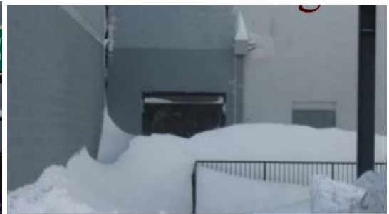
Snow blocked exit.
