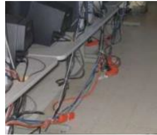
Power bars and extension cords strung together
